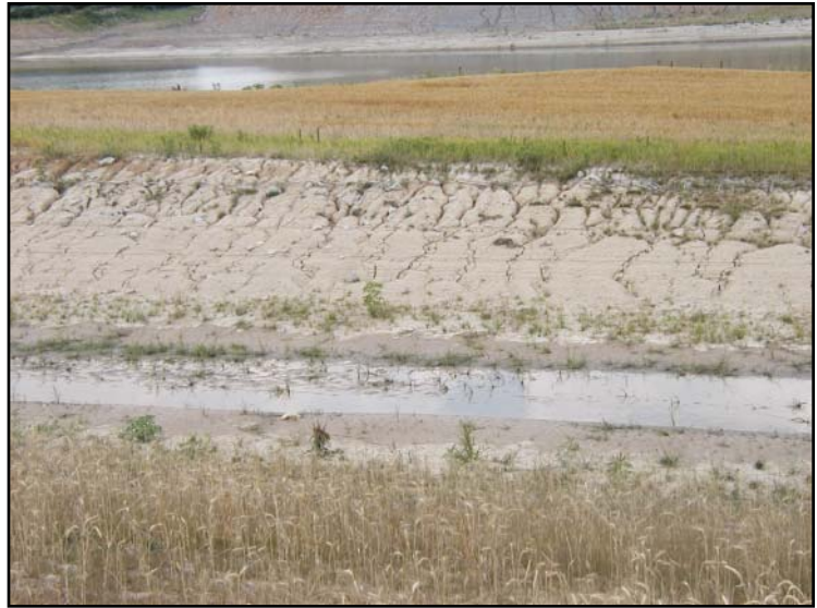
Figure 5.25-3: Eroding Bank on Roadway Construction Project
